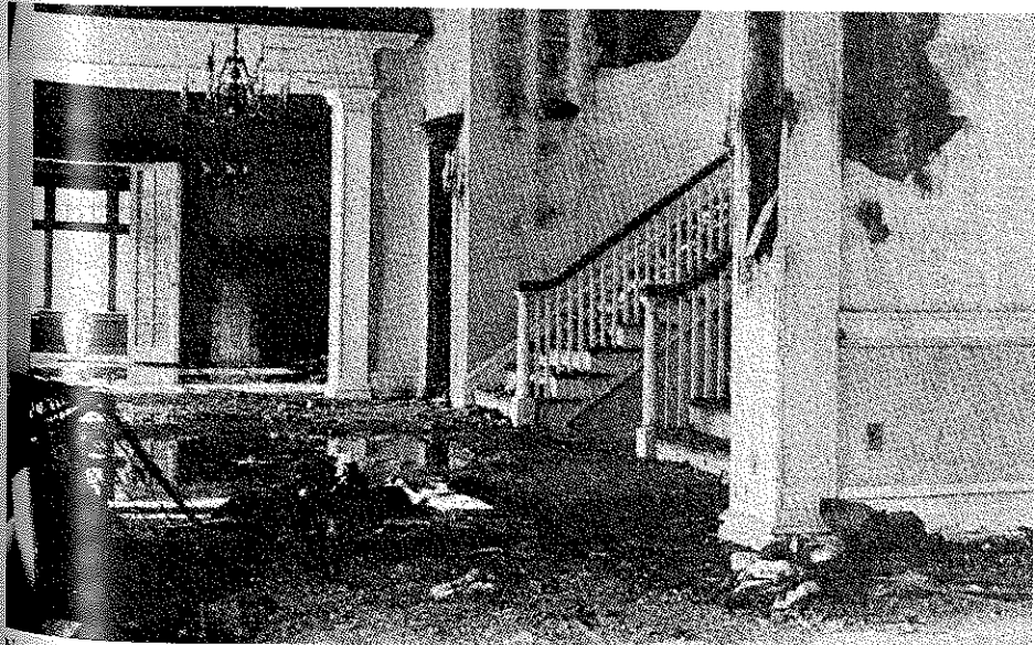
No person was injured in the fire, believed to have been caused by defective wiring in the furnace room.
